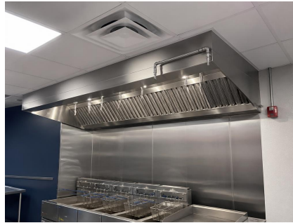
Type I canopy hood with baffle filters and UL300 wet-chemical suppression.
