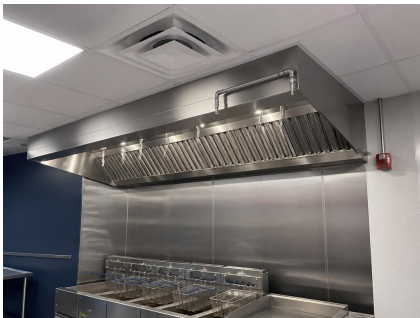
Type I canopy hood with baffle filters and UL300 wet-chemical suppression.
